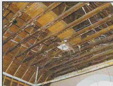
The BCT office ceiling at Finzean Old School ready for repairs after a burst pipe in the roof in January brought down parts of the ceiling.
