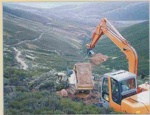
Work in progress on the steep upper section of the Fungle path. Photo © John Addy
