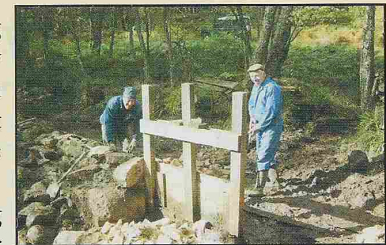
Dave Bulloch and Ian Hector repairing the relief sluice at the Bucket Mill. Photo © John Addy
